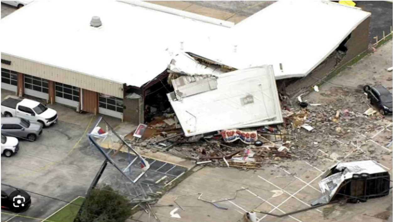
Damage to a large car repair shop in Katy from the EF1 tornado. Courtesy ABC13 Houston
